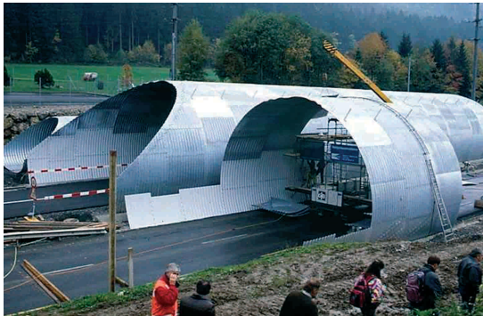
Figure 7.22 - Corrugated steel elements were used for the overpass Schindellegi in Switzerland (40 m wide), which was constructed across an existing road which was widened. This allowed traffic flow along one lane during the whole of the construction phase. (Photo by O. Holzgang)
