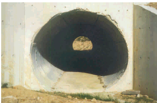
Figure 7.61 - A large culvert made of corrugated steel in Spain designed to allow the drainage of water after heavy rainfall. Filling the bottom with concrete allows it to be used by mammals. (Photo by C. Rosell)
