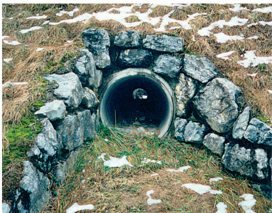
Figure 7.54 - Entrance to an underpass for small animals at the A8 in Switzerland (diameter 1 m). Stone walls, which in this mountain region are a common feature, guide animals to the passage. (Photo by A. Righetti)
