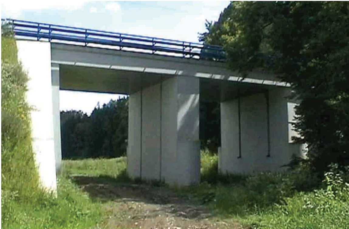
Figure 7.50 - An underpass below a railway line in the Czech Republic. It is combined with an agricultural track which is not tarmacked. Its height also makes it suitable for large mammals. (Photo by J. Dufek)
