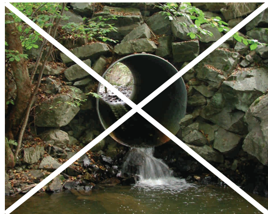
Figure 7.66 - This pipe in Norway was placed too high above the stream. The outfall drop creates a barrier to fish moving upstream. (Photo by B. Iuell)
