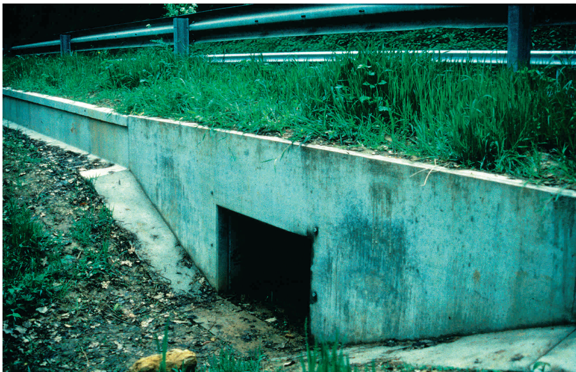
Figure 7.72 - View of a rectangular tunnel in Germany with neatly fitted guiding structures. (Photo by J. Niederstrasser)
