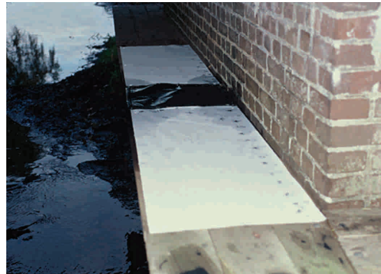
Figure 9.8 - Ink beds are installed on the walkway to allow the passage of small animals such as rodents, shrews or small carnivores to be recorded. (Photo by H. Bekker)
