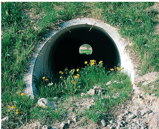
Figure 7.52 - A pipe in Germany (B31neu) designed as passage for small animals. The bottom is filled in with earth, but with a diameter of 1 m it is rather small. (Photo by V. Keller)
