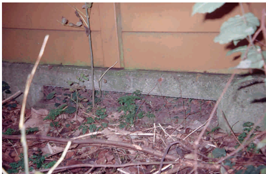
Figure 7.90 - This noise barrier has openings at the bottom to reduce the barrier effect for small animals. (Photo by H. Bekker)
