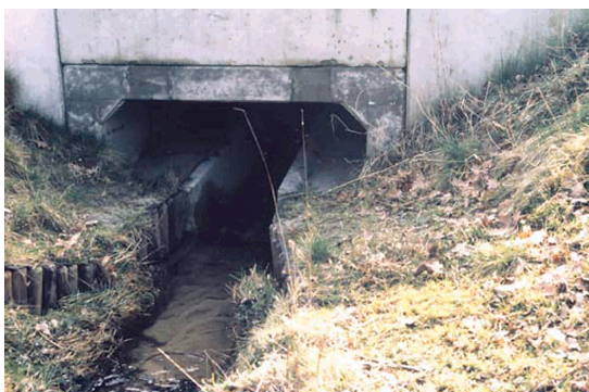
Figure 7.60 - Two prefabricated culverts in the Netherlands (A35, A1) with integrated ledges used by small animals. (Photos by G. Veenbaas and H. Bekker)
